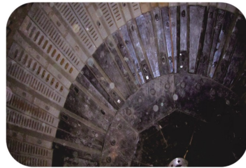
D.E. rubber liners on \Phi 10.37 \times 5.19\text{m} SAG mill
